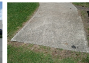
Footpath terminating abruptly
